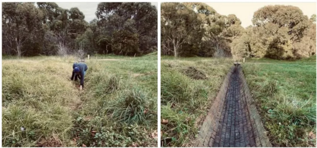
Source 3. Before and after the clearing of the Victorian swale drain below the old Asylum (now a gated community).
